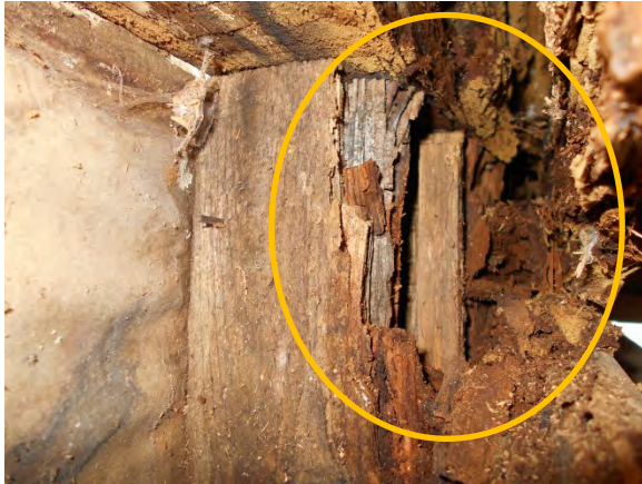
Image 1.16 Deteriorated exterior wall at kitchen
