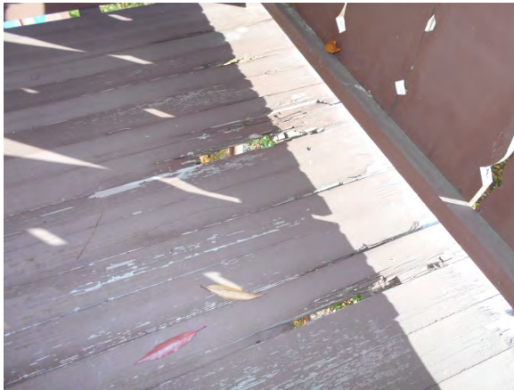
Image 1.11 View of the deteriorated balcony deck at the east
