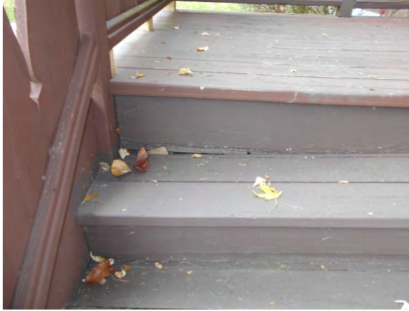
Image 1.21 Deteriorated front porch steps
